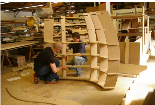
Figure 5. Shelves, Design and Engineering: Ivo Vrouwe. An example of Phase 1; Volume patterning reframed into a surface-active system by the use of wood.
